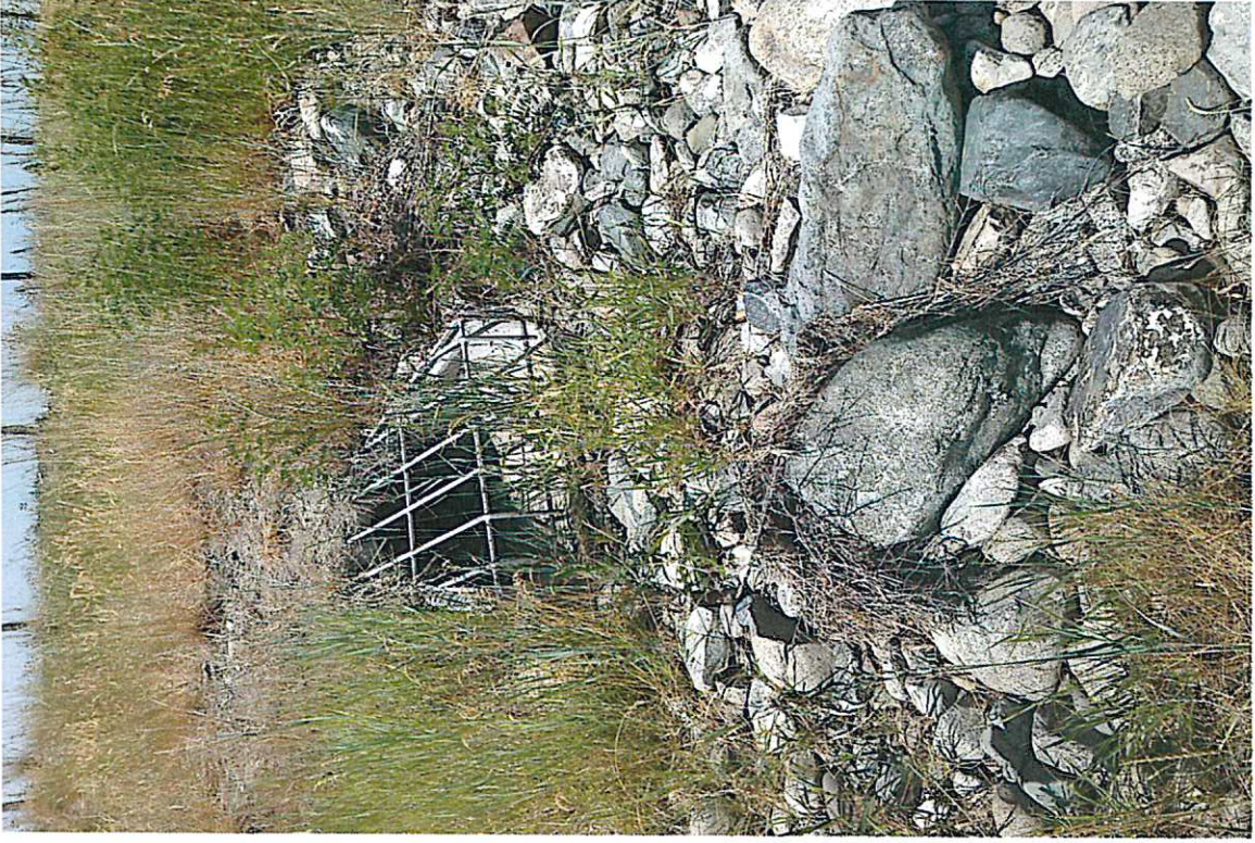
OUTFALL 4 - FERGUSONS POND INLET
