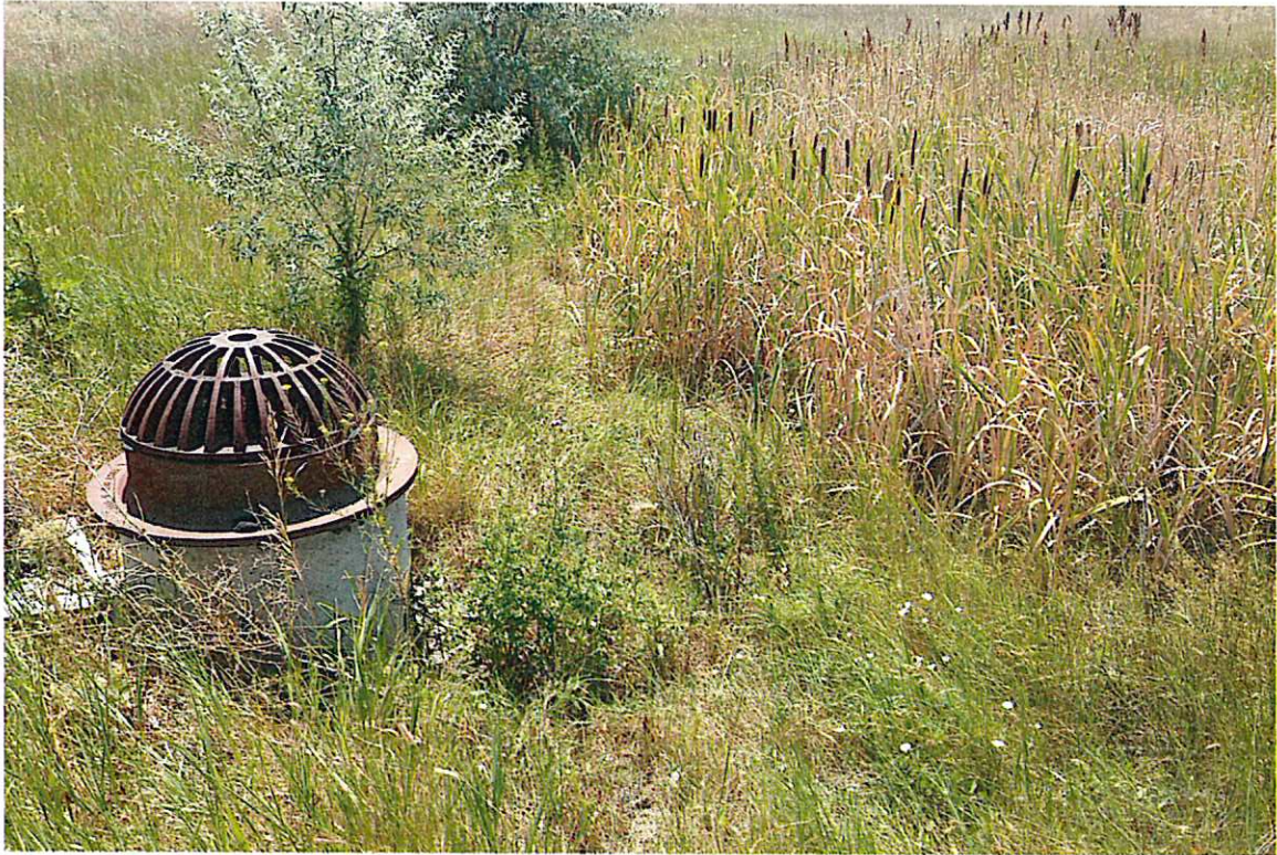
OUTFALL 5 - NORTH POND OUTLET
