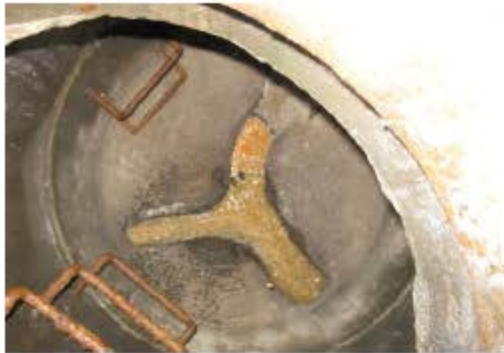
Grease clog in sewer.
