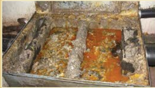
GRD too full of FOG and not maintained properly.
