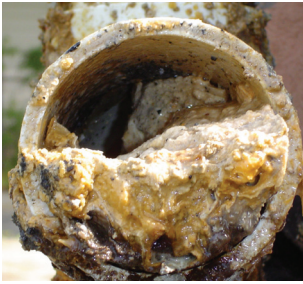
Grease clog inside a pipe.
