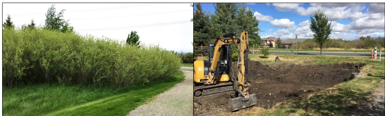
Figure 5.7-6. Detention Basin Deferred Maintenance
