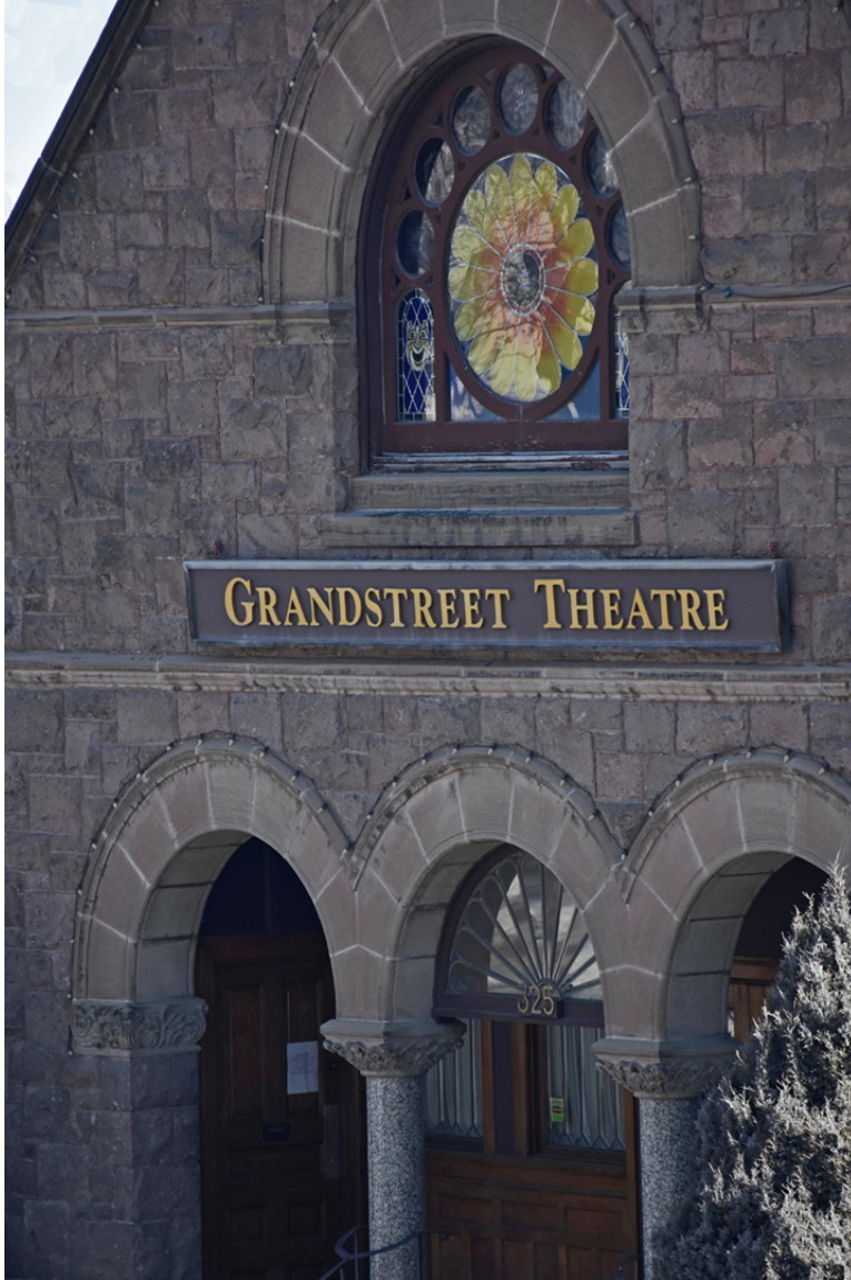
Figure 8.02 – Though many structures were razed during "urban renewal" efforts in the 60s, survivors, such as the Grandstreet Theatre, provide significant aesthetic, functional and cultural value to Helena. (Image: SCJ Alliance, Inc.)
